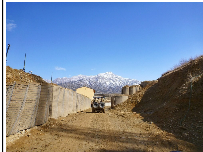
HESCO walls lining the Combat Outpost in eastern Afghanistan. Courtesy of Jackie Munn
